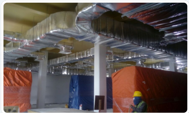
HVAC Ducting Sys. inside RO Elect. Building
